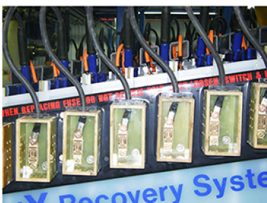
Sealed DC Fuse Boxes for Each Individual Chamber with Plastisol Encapsulated Bus Bar
